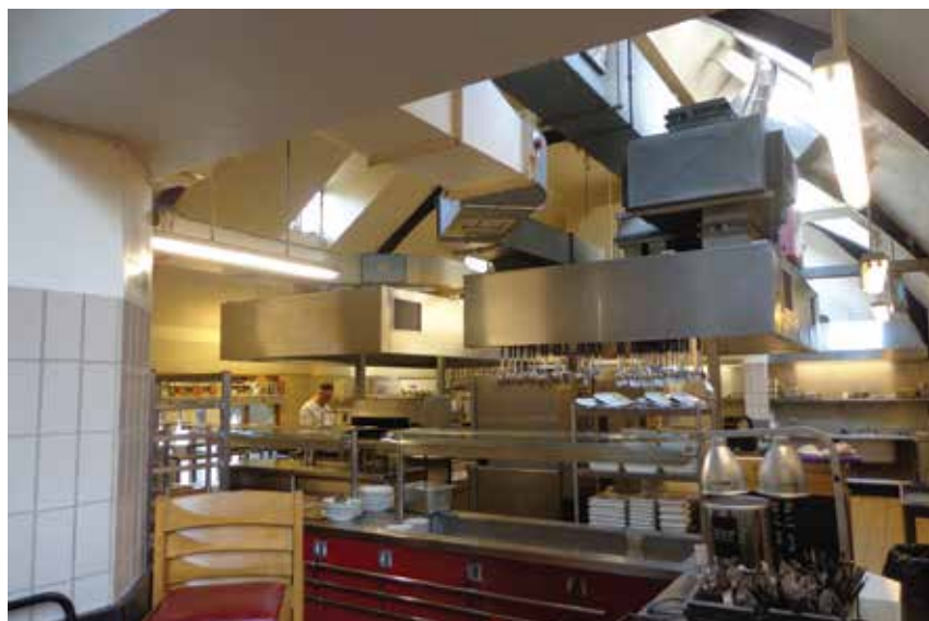
The existing servery and kitchen. This space is to be reconfigured as a free-flow servery. All extract ductwork will be removed. Compare this picture with the lower image on p. 12
