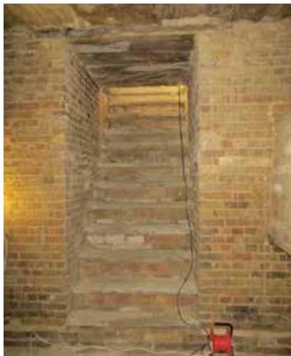
Left, the extremely steep steps up to the chapel Right, end of a cast iron joist supporting York stone slabs
